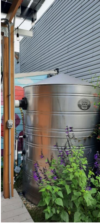
Figure 7.4: Stored rain water to be used for garden irrigation.
