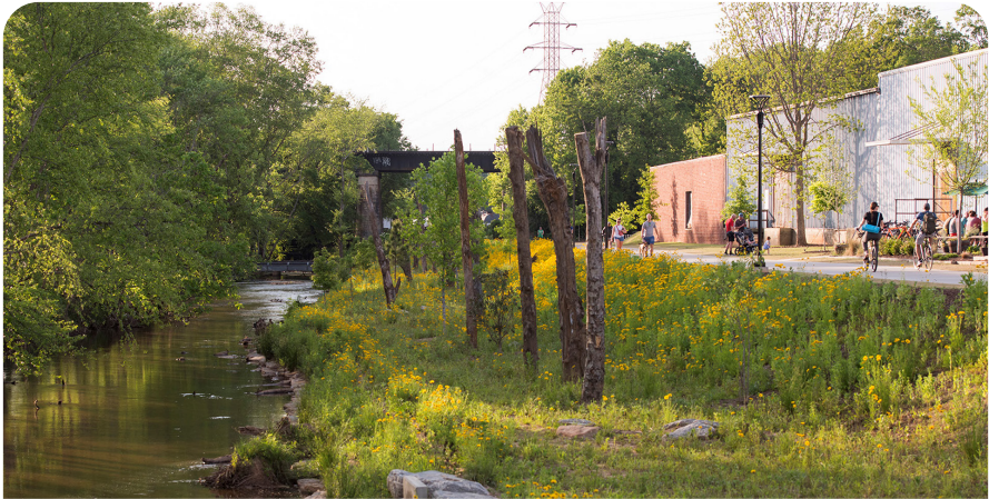
Above image: Stream restoration case study project at Unity Park, Greenville, SC.
