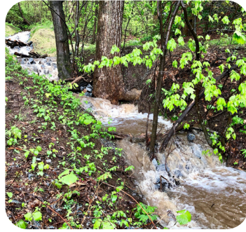
(Above) Stream restoration project at Givens Estate a 200 - acre retirement community in Asheville, North Carolina.
