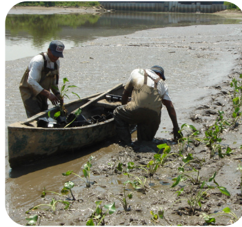
(Above) Anacostia Wetland Restoration – Planting freshwater tidal wetland plants along the shoreline of the Anacostia River in Washington D.C., to enhance aquatic habitat and improve water quality.
