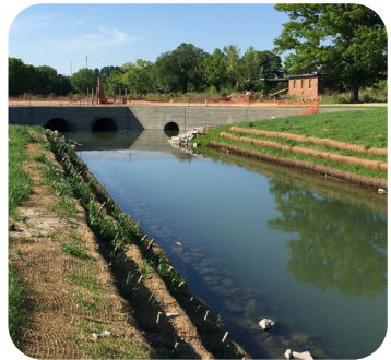
(Above) Daylighting and stream restoration of Smith Branch in Columbia, South Carolina. Of the nearly 3,000 linear feet of stream located at the park, 2,000 had been piped underground since the 1950's. RDE's stream daylighting design restored the stream to the open air and revitalized the floodplain, now a key attraction of the public park.
